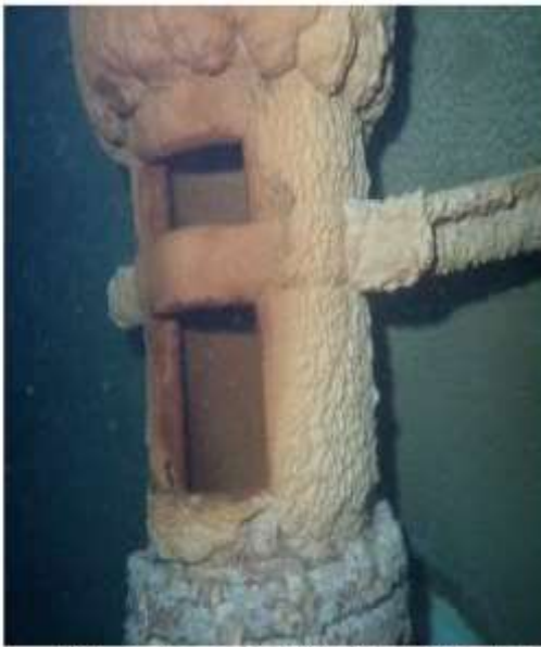
16" Inside Diameter Pipe With A Cutout, Moderate To Heavy Calcified Lime And Corrosion
