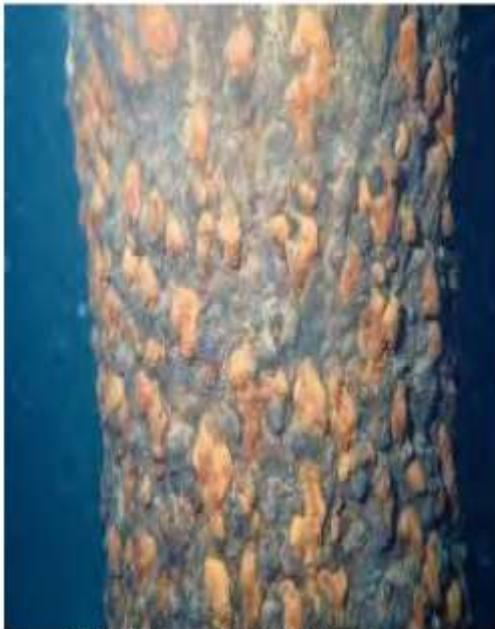
16" Inside Diameter Pipe With Corrosion
